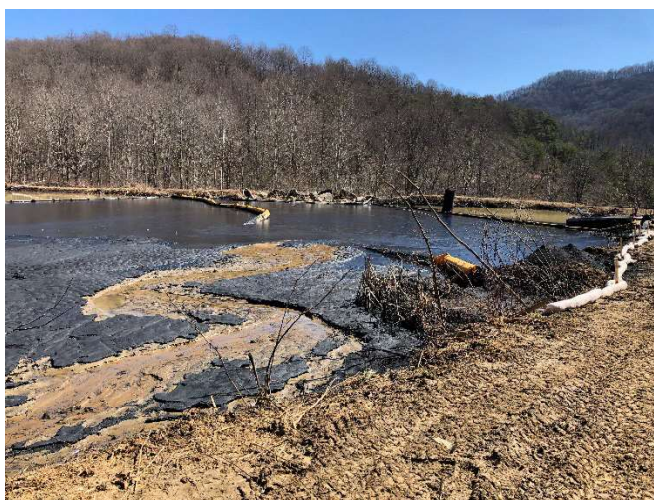
1 Heavy Sediment fills the pond to the surface on the south end
